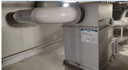
Busan OO Non-Point Source Pollution Reduction Facility
