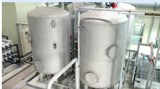
OO Food Factory Industrial Water Treatment Plant
