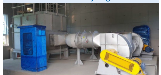
Seoul OO Water Recycling Center
