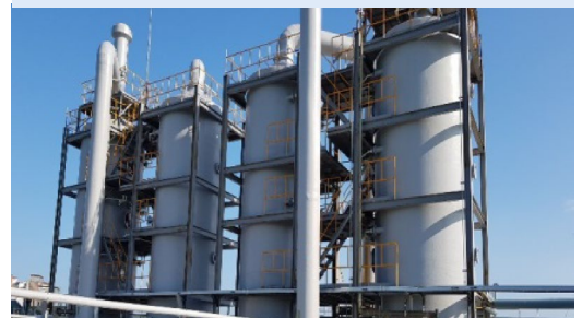
Busan OO Leachate Treatment Plant
