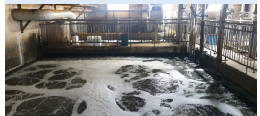
Busan OO Leachate Treatment Plant
